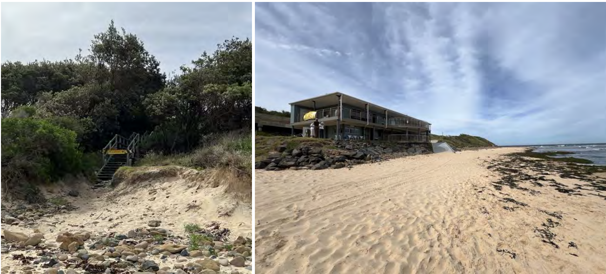
Figure 3.38 Sandon Point SLSC - reduced beach access (left) and exposure/proximity to wave overtopping (right)
